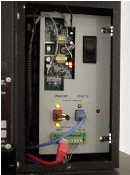
Telephone Audio Interface with test plug installed in the RED or Window Lane
